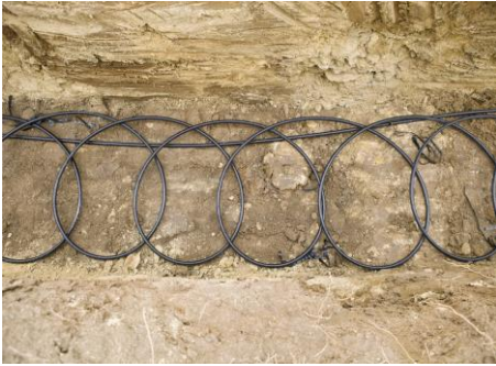
One of the barriers to wider adoption of geothermal heating and cooling has been the cost of ground loops.
